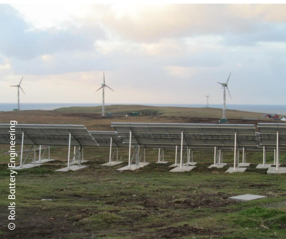
Fair Isle's lead battery microgrid harnesses renewable energy from wind and solar sources.
